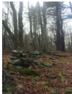
Figure 2. Photograph of the ice storm damage site looking at the rock wall from the pasture side.
